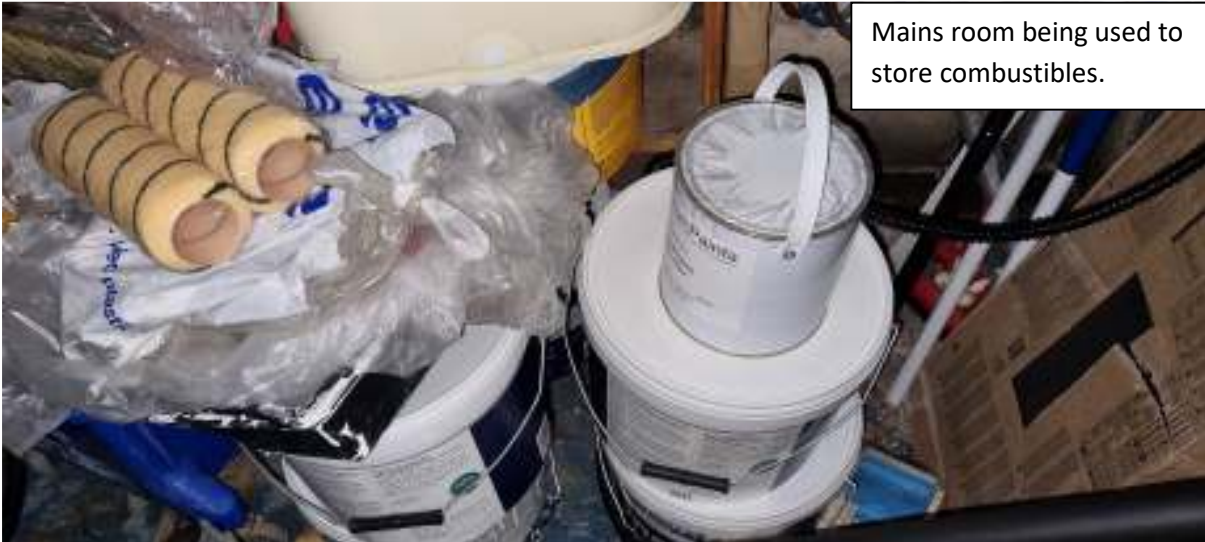
Mains room being used to store combustibles.
