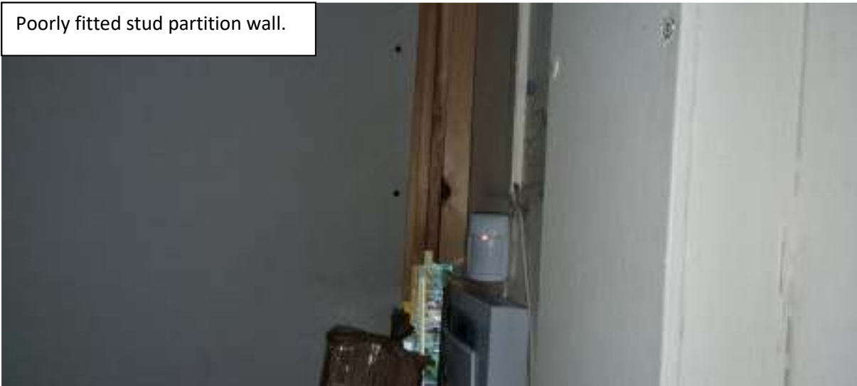
Poorly fitted stud partition wall which has gaps into the new kitchen with no working fire detection nor fire compartmentation. If a fire started in the kitchen it would spread quickly through the building.
