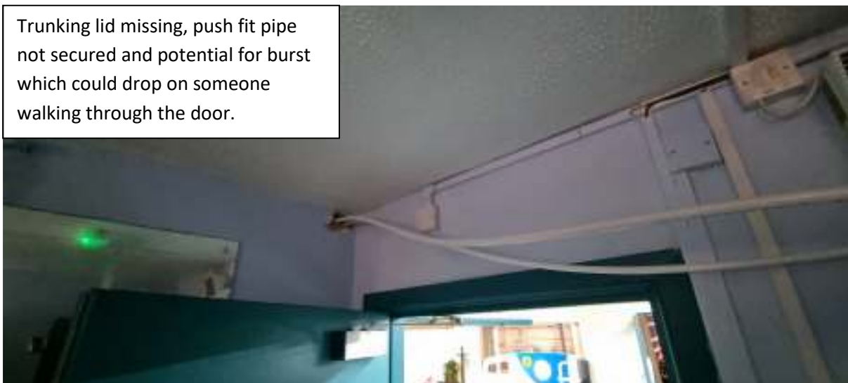
Heating circuit push fit pipes poorly installed not secured and liable to leaking causing further building damage.
