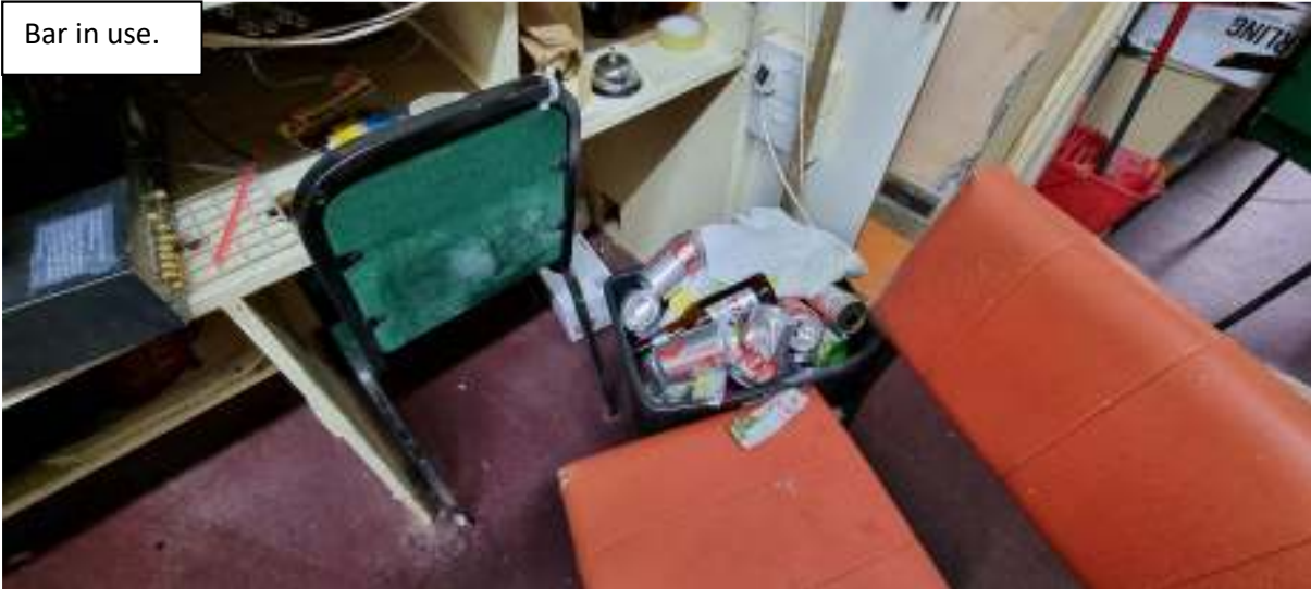
Cables not being run correctly no protection.
