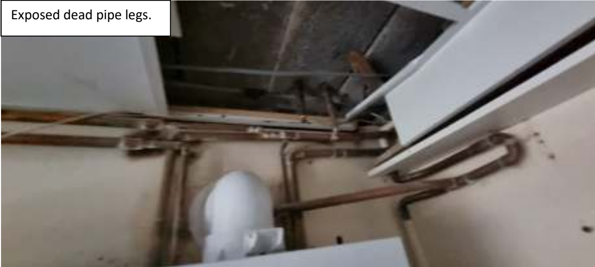
Electrocution risk here.
