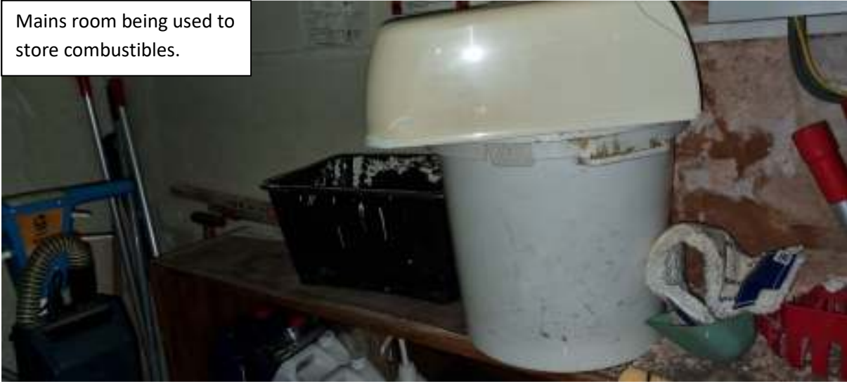
Mains room being used to store combustibles.
